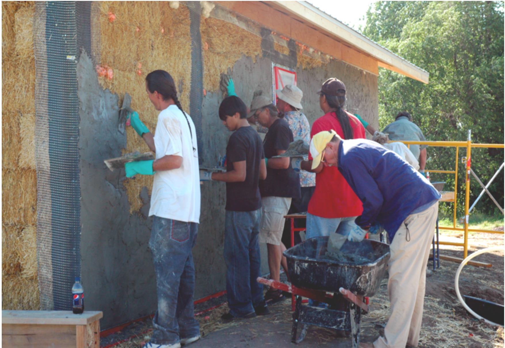
COUP SGU Buffalo Lodge Straw Bale Building Exterior Plastering: Portland-Lime plaster mix applied as a rough or scratch coat.
