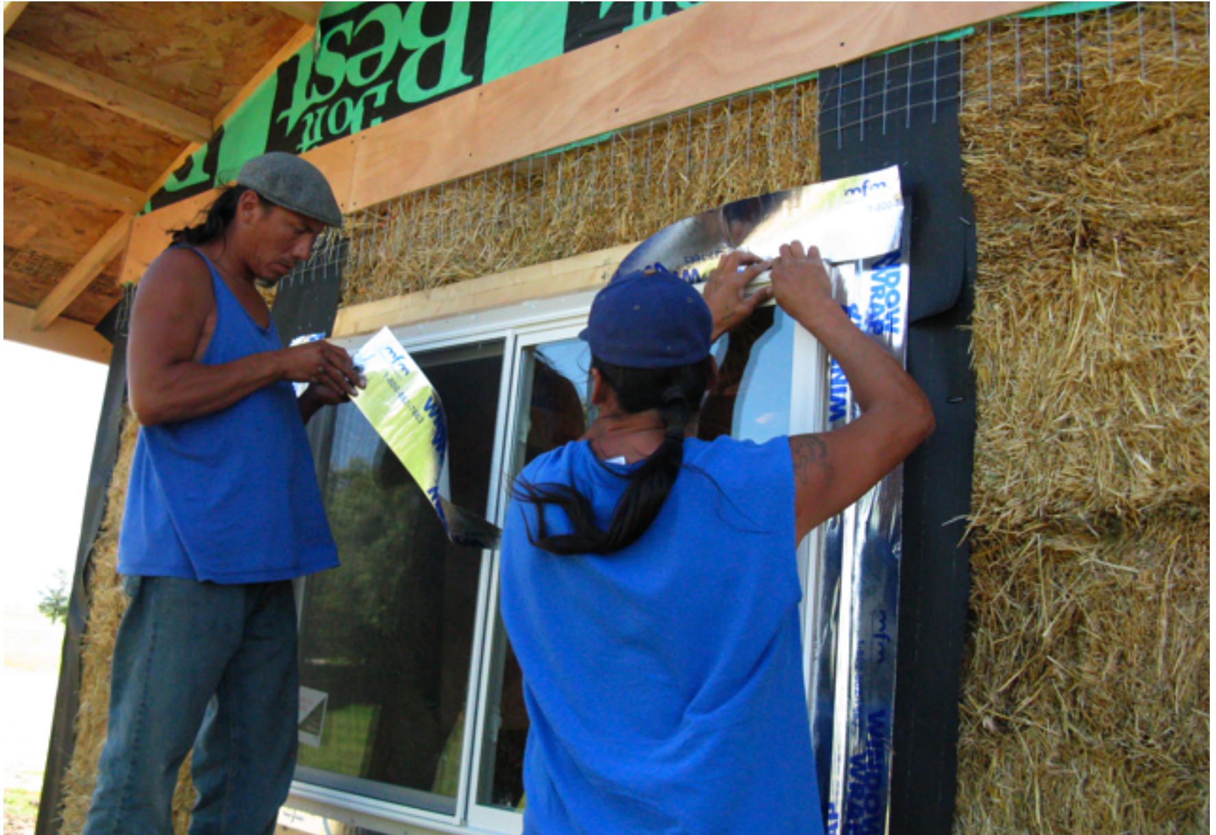
COUP SGU Buffalo Lodge Straw Bale Building Window Wrap Installation: Used to seal out water leakage along the window frame.
